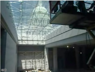
The underground visitor center, seen here under construction, has skylights allowing views of the Capitol.
